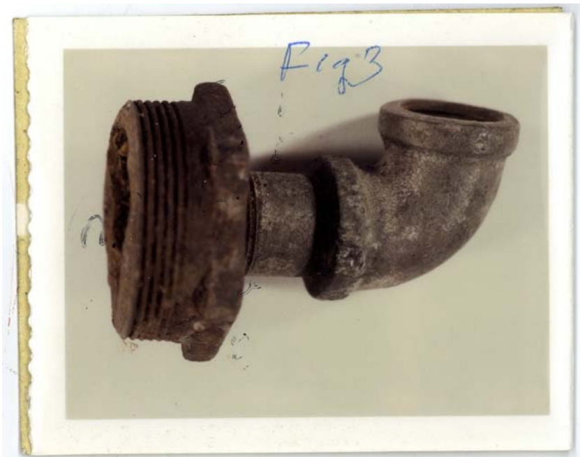
Figure 3: Failed bushing, from the other side.
