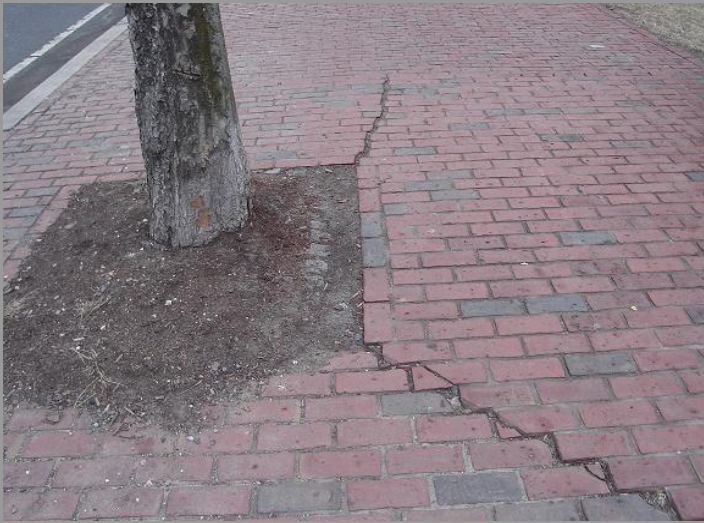
Figure 13: Photo (4) Roots cracking sidewalk
