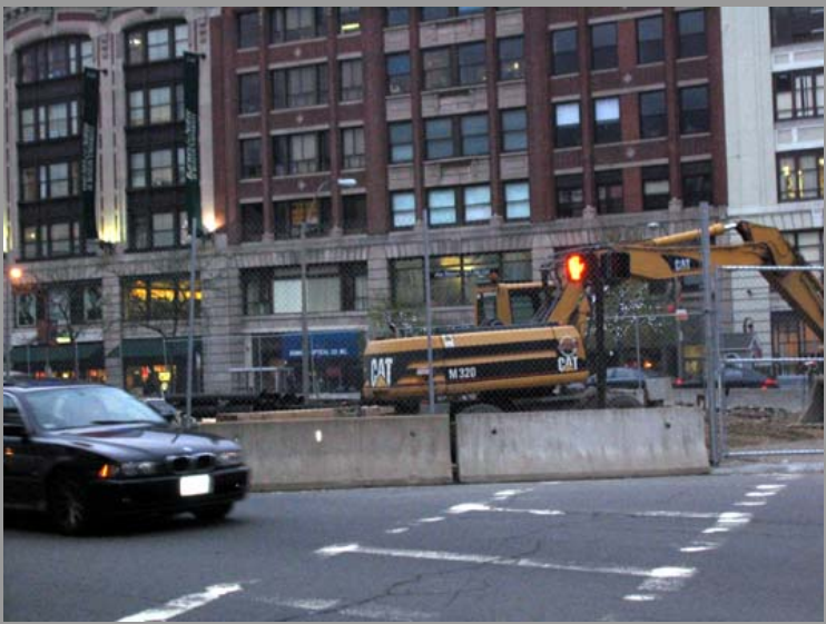
Figure 18: Construction on Commonwealth Avenue where the Bus Center used to be located.
