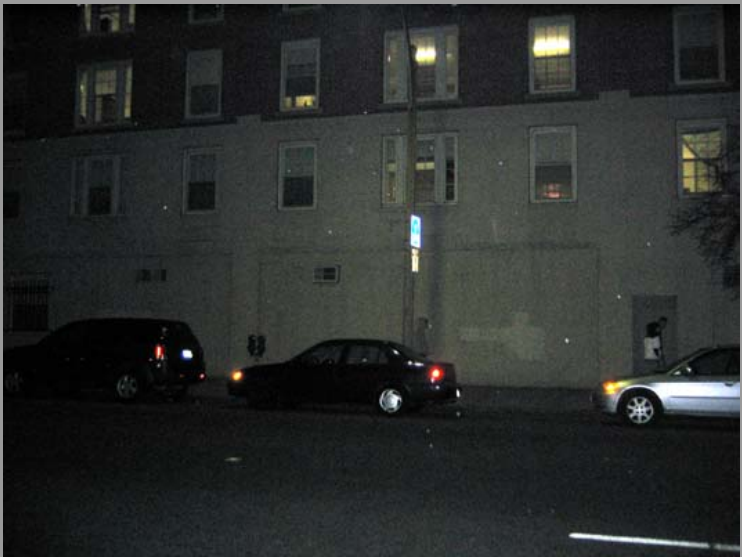
Figure 8: Discoloration on the wall which once house the storefront windows.
