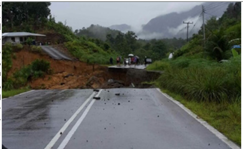
Figure 22. Road off of Jalan Puncak Borneo (near Bengoh Dam) caved in after heavy rains. © Borneo Post. All rights reserved. This content is excluded from our Creative Commons license. For more information, see http://ocw.mit.edu/help/faq-fair-use/
