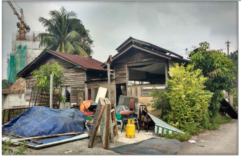
Figure 13. A house in Kampung Chubadak Tambahan designated for demolition for the private housing project. Photo Credit: Vishnu Prasad, 2016
